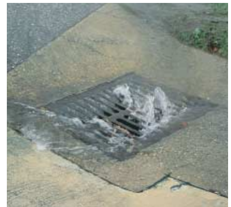
Stormwater runoff can easily overwhelm existing drainage facilities
